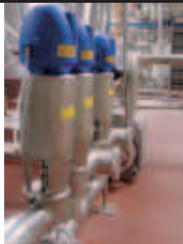
Unique MixProof valves and ThinkTop controllers from Alfa Laval comprise the heart of the flow system at the Gay Lea plant in Guelph, Ont.
